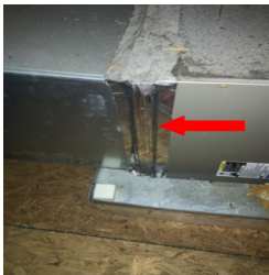
The small access cover on the intake of the air handler was sealed and could not be removed.
