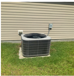
HVAC System Heat Pump
