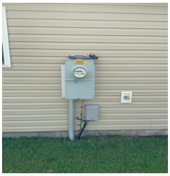
Electrical Service Entry
