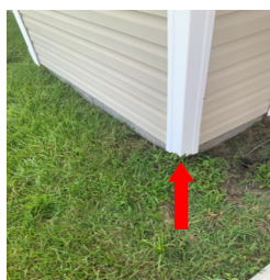
Corner posts for the exterior wall cladding are damaged.
