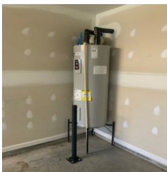
Electric Water Heater in the Garage
