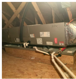
HVAC System Air Handler
