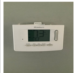
The heat pump and air handler HVAC system failed to cool the home during the inspection.
