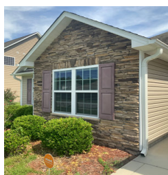
Adhered masonry stone veneer exterior wall cladding is installed on this house.
